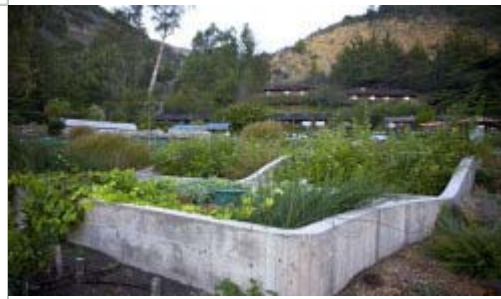
This "tidal-flow wetland" Living Machine treats wastewater from the laundry and lodging facilities at the Esalen Institute in Big Sur, California, for use in irrigation and aquifer recharge.
